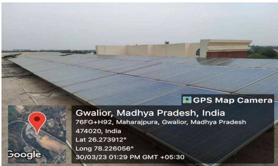
Solar Power Plant
